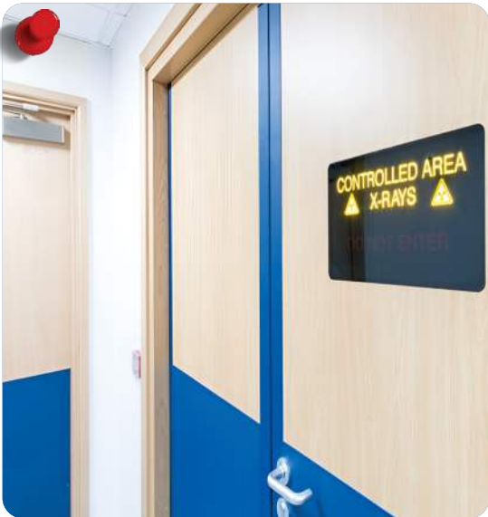
FLUSH MOUNTED DOOR WARNING LIGHTS
